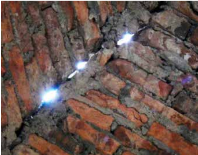
Figure 11. Cracks in the caps of the Santa Lucia Temple's dome Source: photograph by authors.
